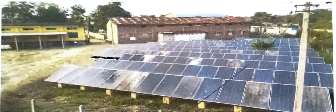
Fig: 2 Solar Power Plants
